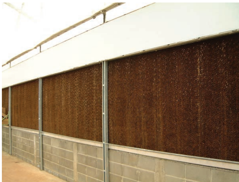
Figure 1. Outside air that is pulled through a well-designed and maintained pad system by exhaust fans can effectively cool a greenhouse.
